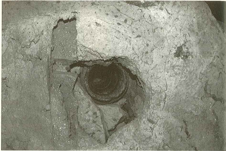
Fig. 41 - The pipe on the vault of the hypogeum and the white marble slab from its earlier phase.
